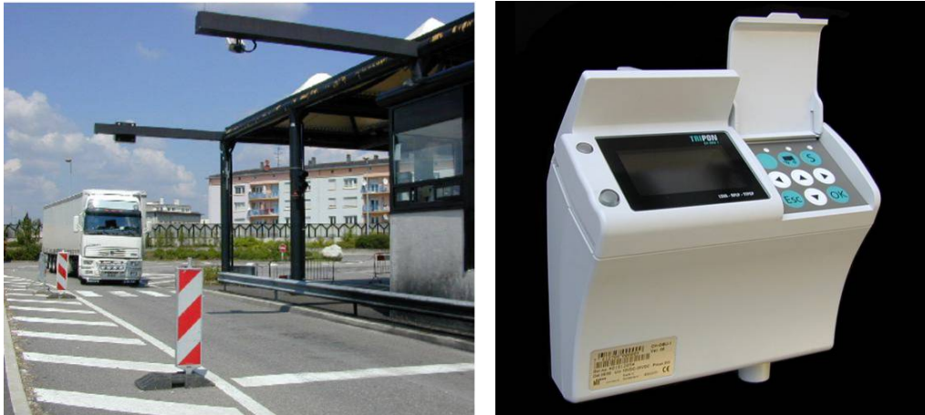
Figure 21: A Swiss Border station equipped with DSRC beacon and the Swiss OBU
